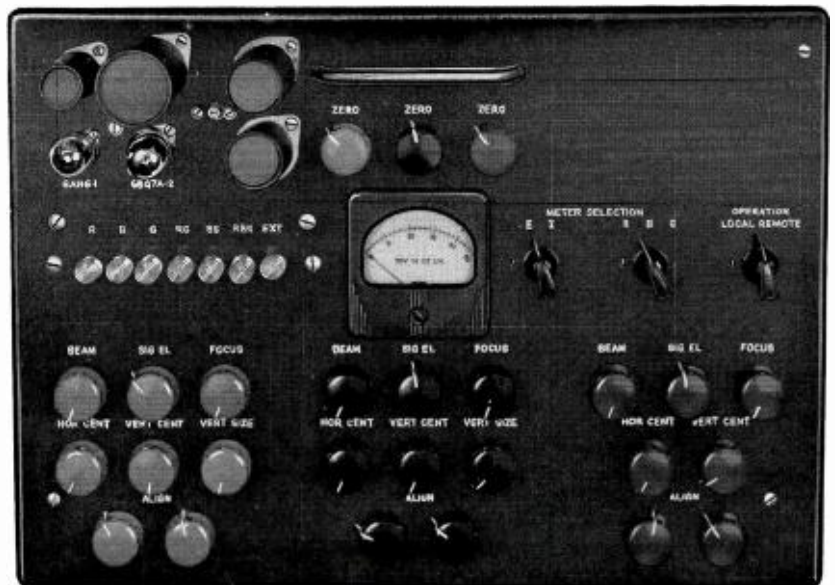
FIG. 11. Local control panel.
